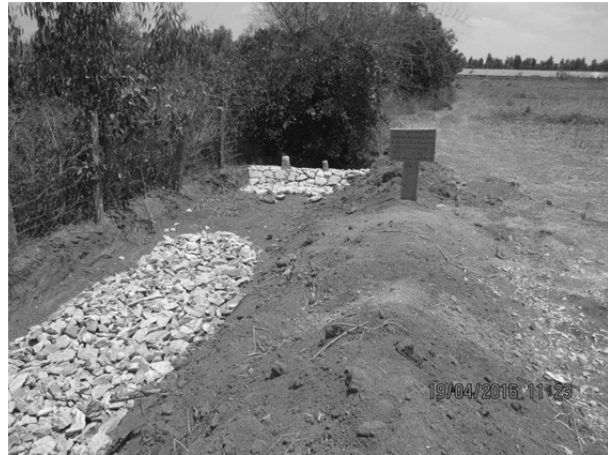
Fig. 7. Boulder check & recharge well
